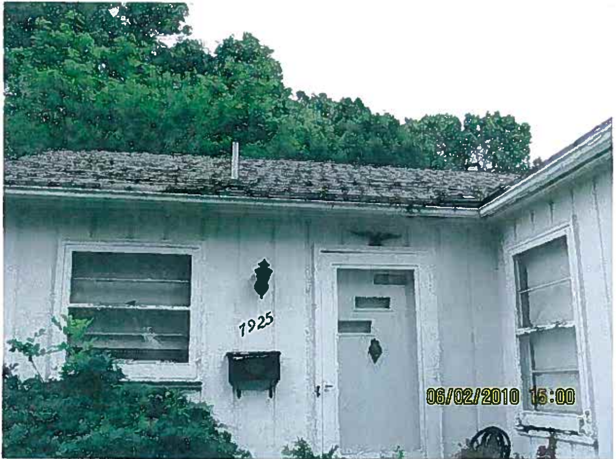
Front door, windows, debris and other roof area
