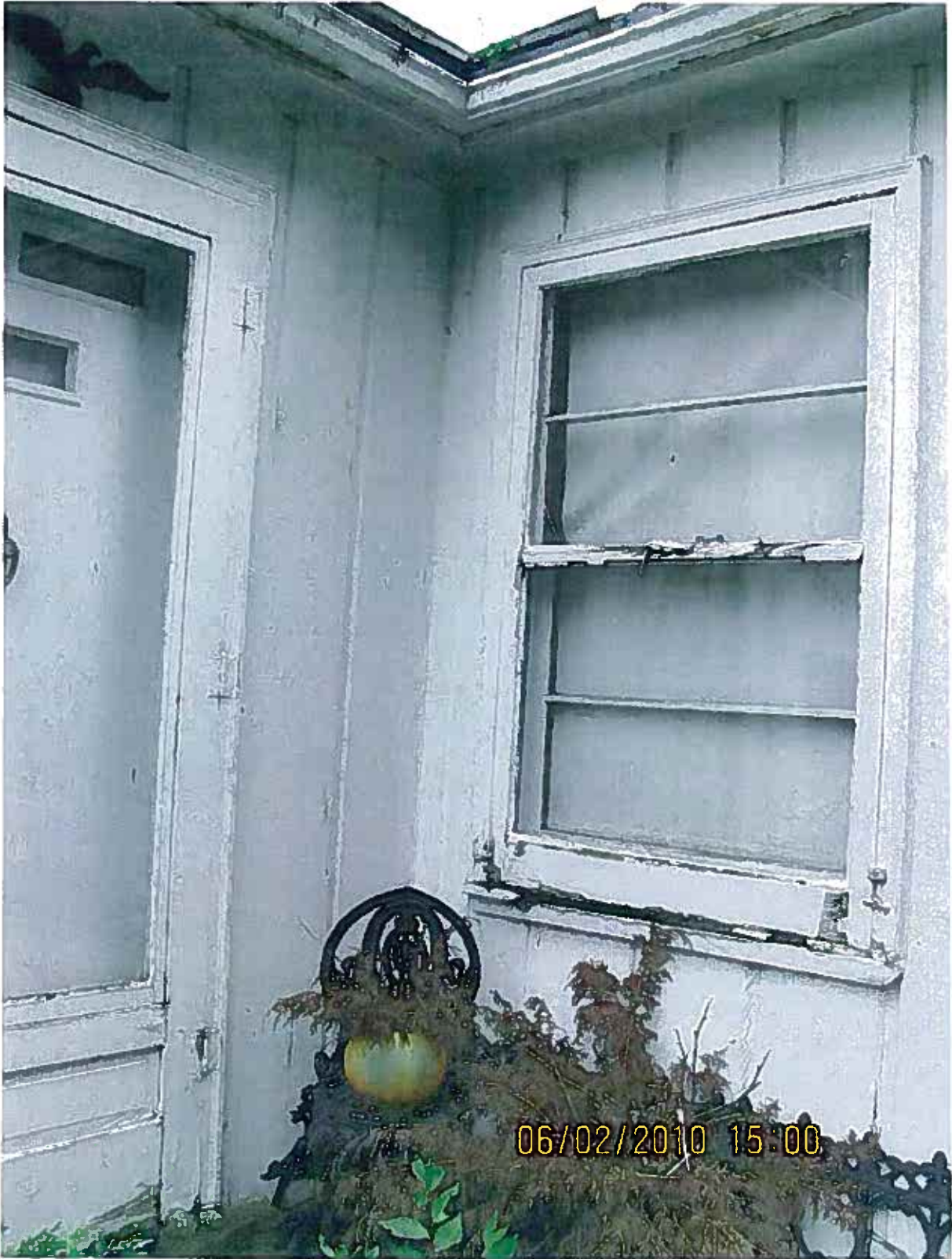
Front door, windows, debris and other roof area
