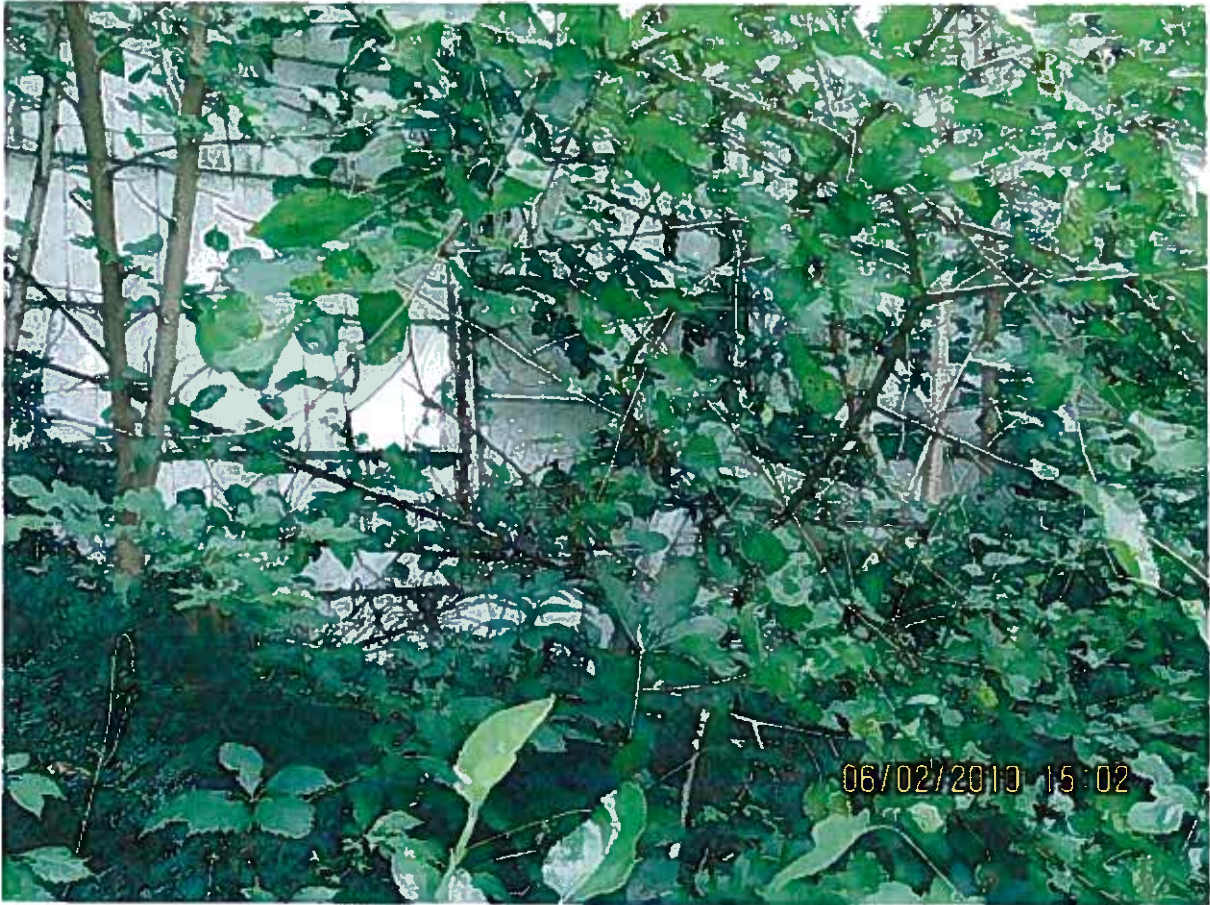
South side of house, overgrown vegetation and storm window fallen out
