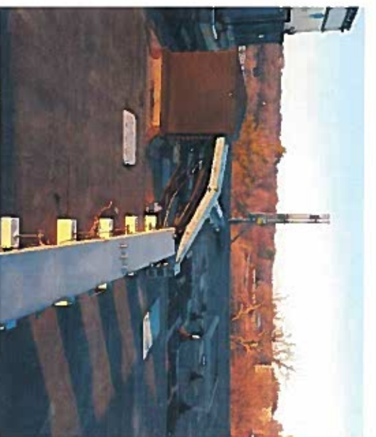
7 LESSEE COAX ROUTE AT ROOF HATCH PENETRATION
