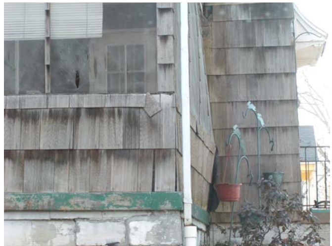
Peeling paint on porch trim
