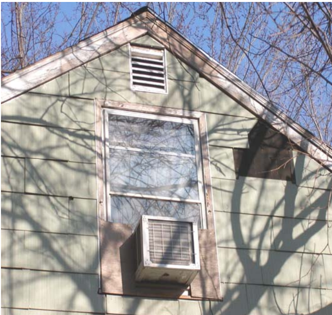
Missing Shingles and peeling paint
