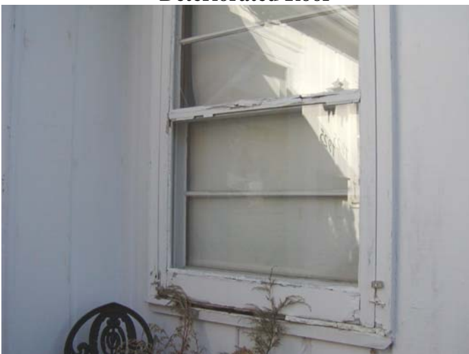
Peeling paint, rotting wood
