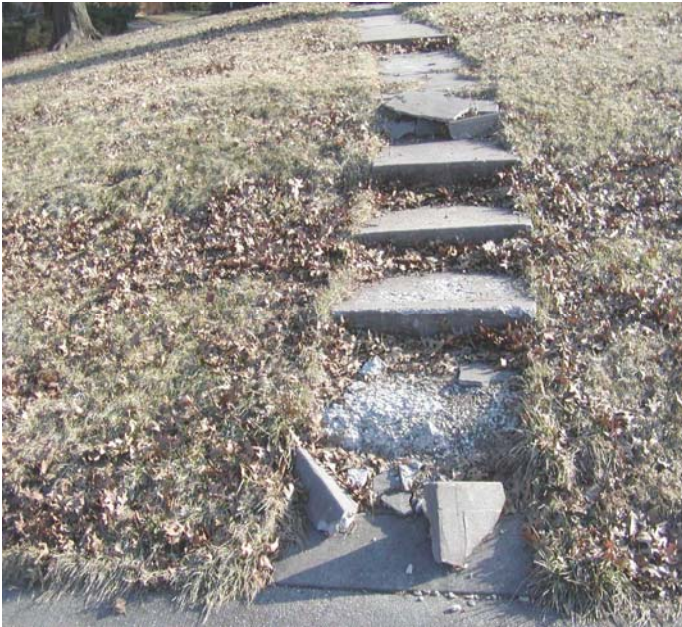
Broken and deteriorated front walkway
