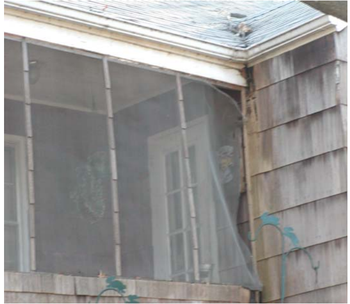
Torn screen on front of porch
