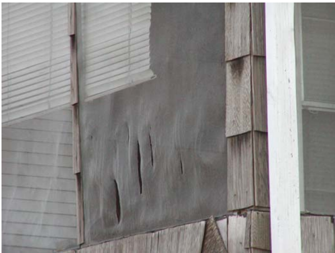
Torn screen on side of porch
