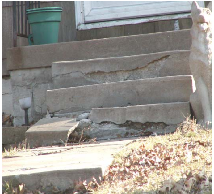
Broken and deteriorated front steps
