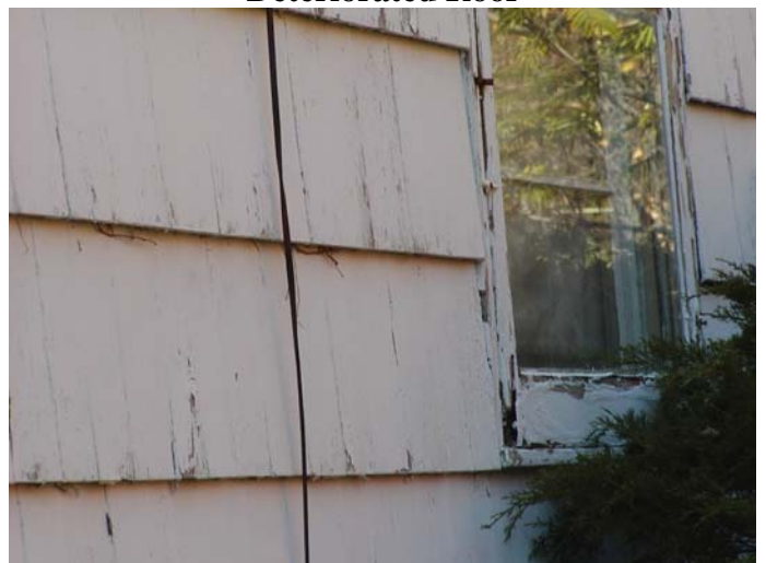
Peeling paint, rotting wood
