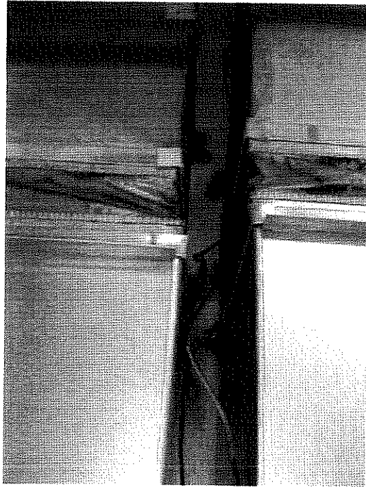
Photo No. 3 View of wall behind ductwork in the mechanical room. Note: Visible fungal growth and debris from inside supply duct that has impacted on the wall.
