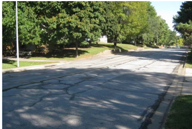
4 Through Lanes, Non ADA Compliant Sidewalk
