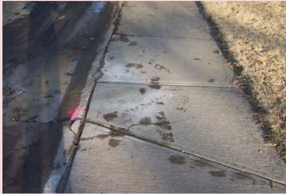
The Concrete Repair program sidewalk replacement focuses on a work area annually. CONC2017 will be in district 31.
