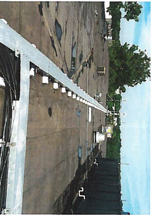
6 LESSEE COAX CABLE TRAY ON ROOF
