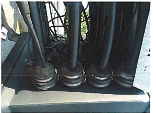
4 LESSEE COAX ROUTE AT DOGHOUSE ON ROOF
