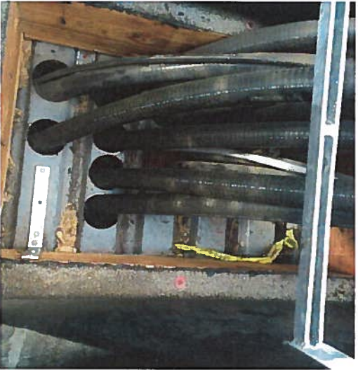
5 LESSEE COAX ROUTE AT ROOF HATCH PENETRATION
