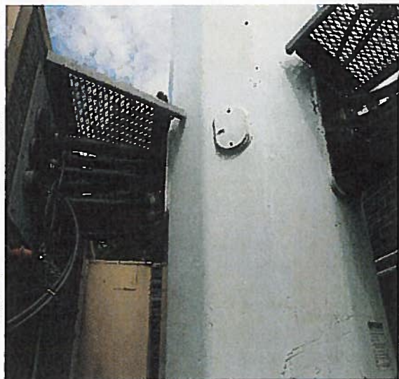
2 LESSEE COAX ROUTE ON TOWER
