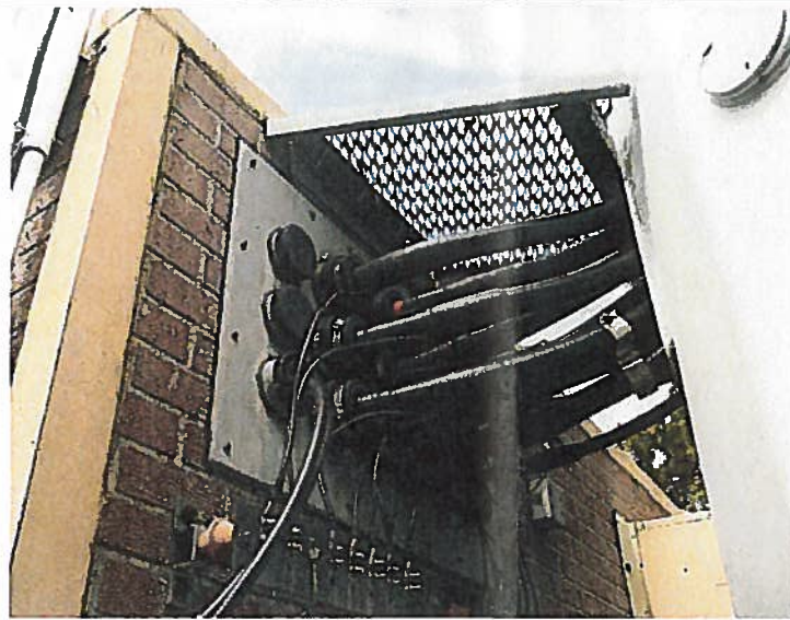
2 LESSEE COAX ROUTE ON ICE BRIDGE
