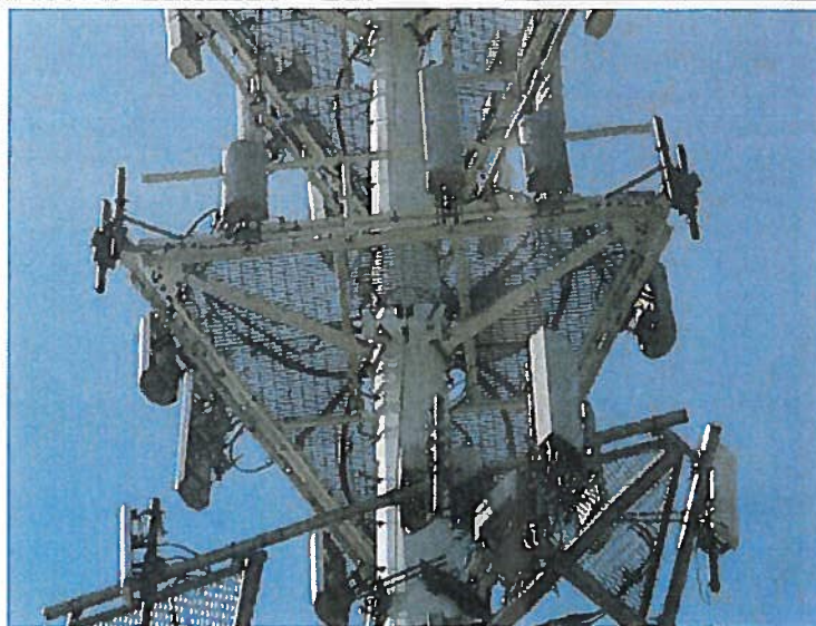
3 LESSEE COAX ROUTE @ TOP
