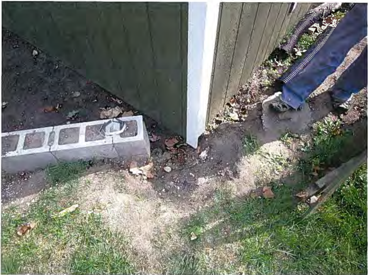
Corner of Garage in Relation to the Retaining Wall
