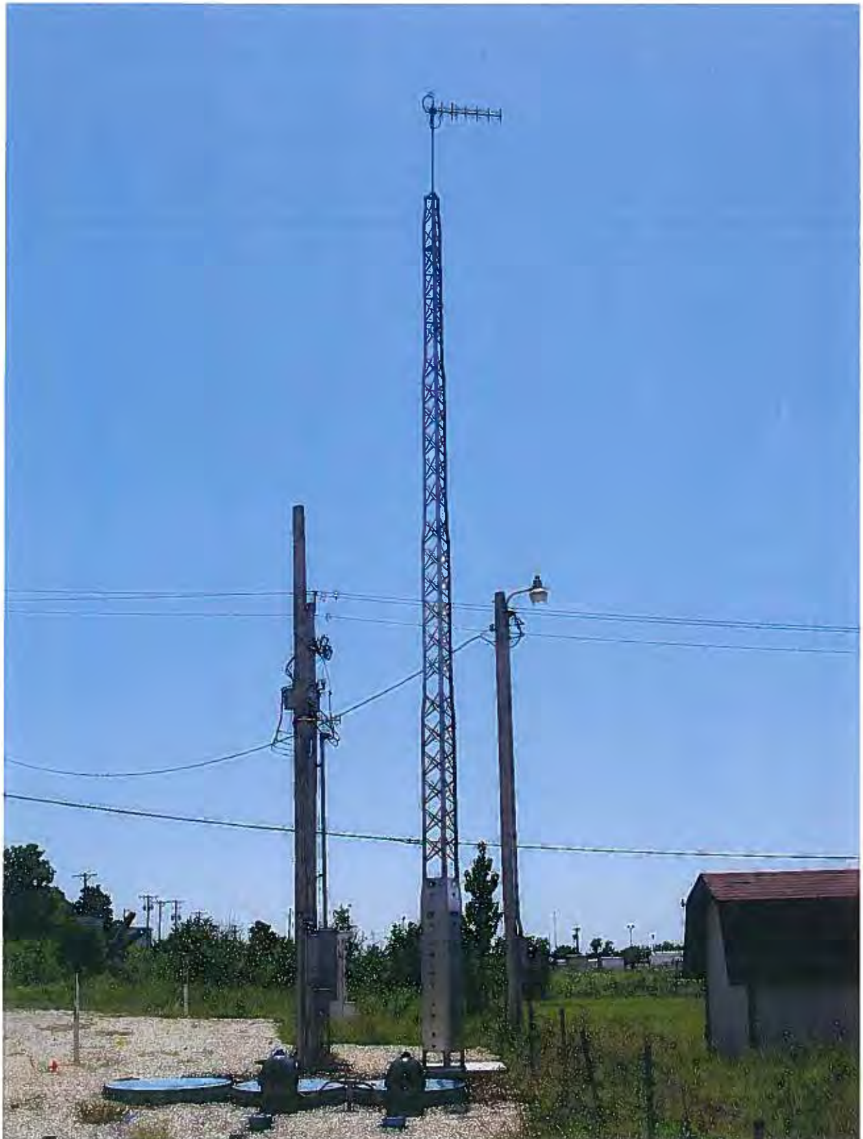
Example of a Tripod, lattice style antenna tower.
