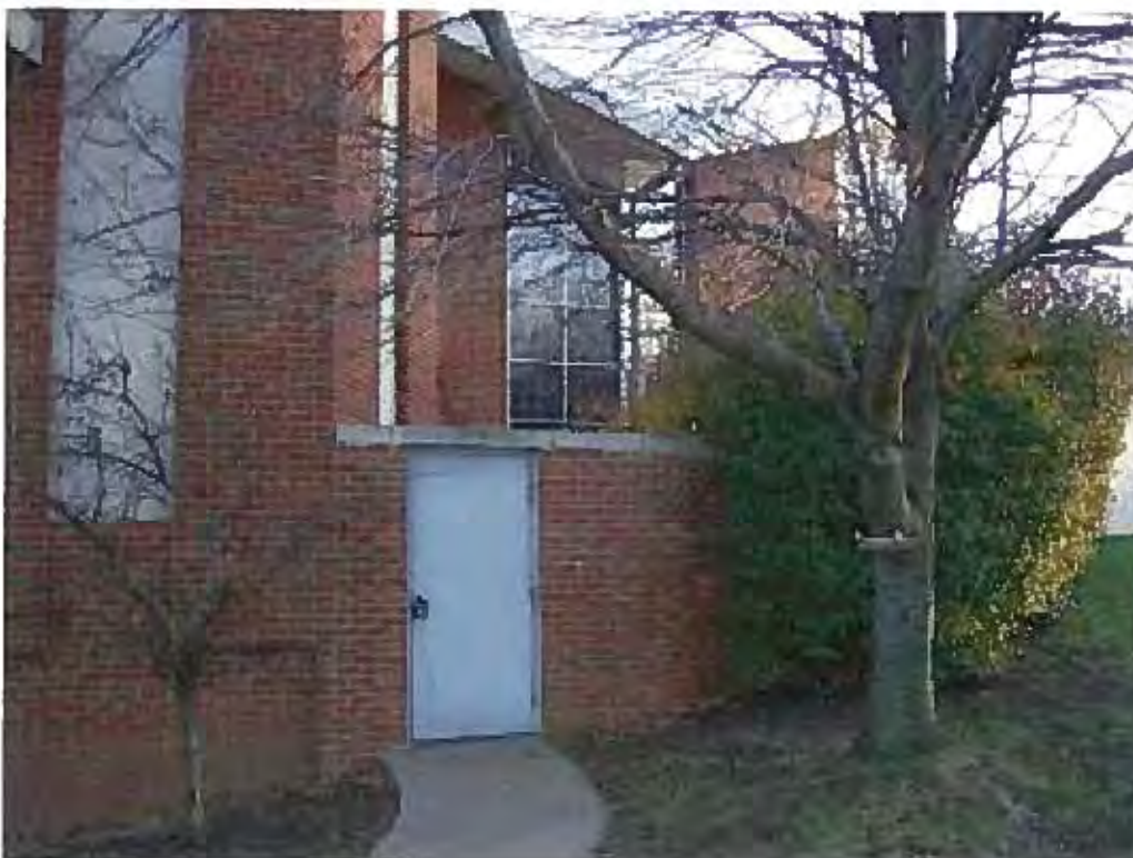
Equipment Compound (St. Anns)
