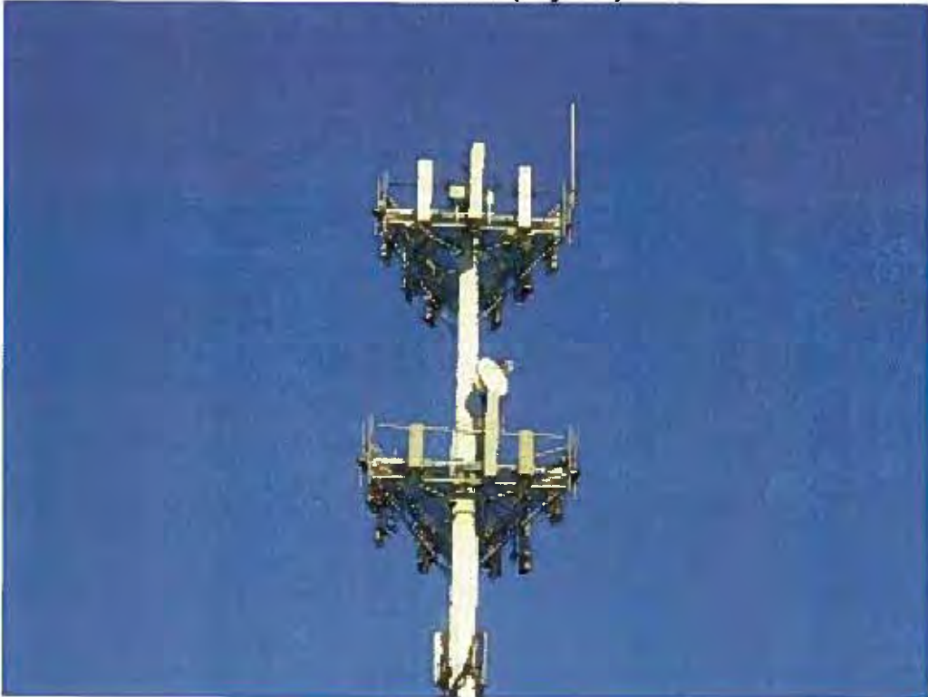
Antennas (City Hall)
