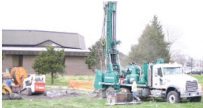
Geothermal installation at Pittsburg State University
