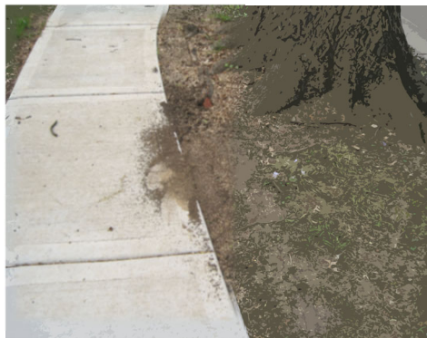
The Concrete Repair program focuses on a work area annually to repair curb/gutter and sidewalks.
