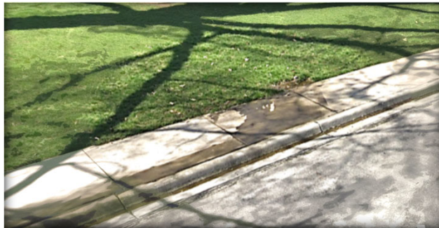
Eliminating nuisance sump pump discharge can minimize infrastructure repairs.
