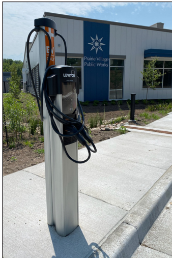
Electric vehicle charging station
