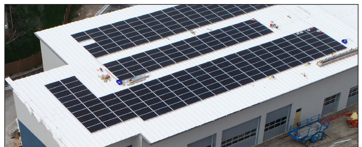
Solar panels mounted on the roof are expected to supply just over 50% of the building's power needs.
