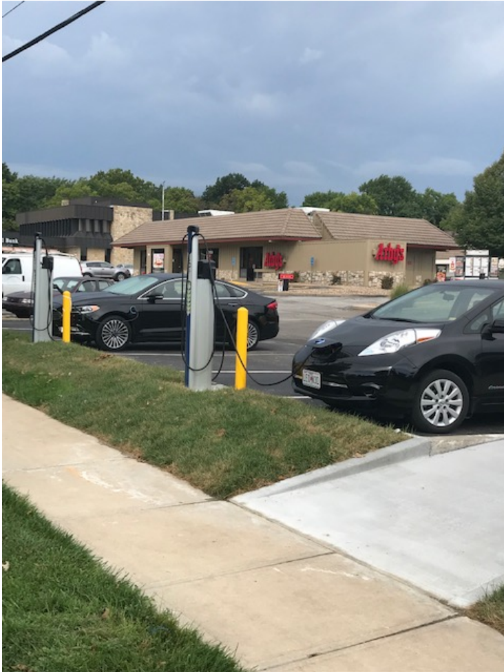
Corinth Square EVSE Charging Stations
