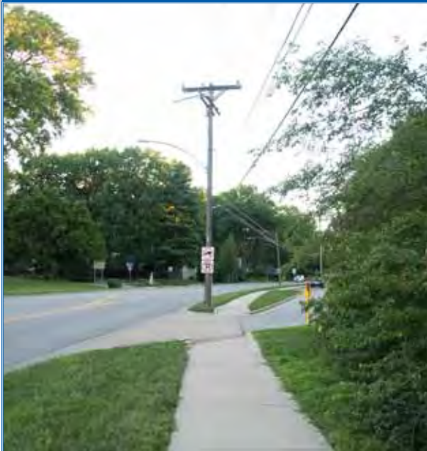
Figure 6. Mission Road utility poles and power lines
