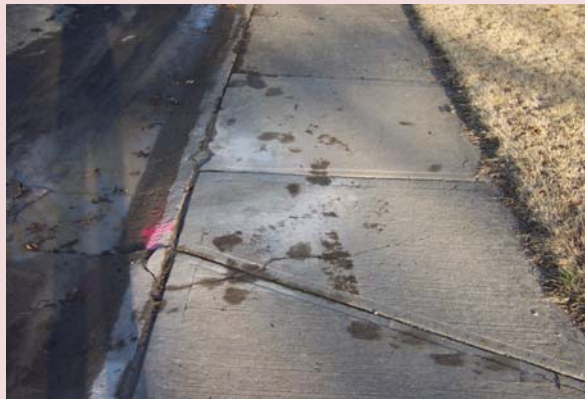
The Concrete Repair program sidewalk replacement focuses on a work area annually. CONC2019 will be in Districts 12 and 13.
